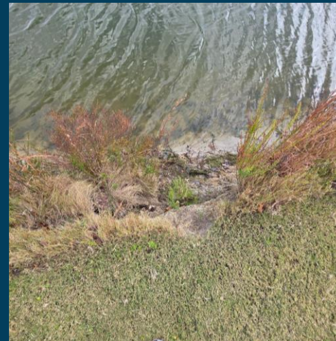
Lake Bank Erosion near lake #3
