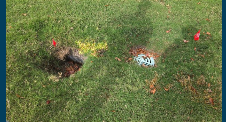
Sinkhole near the 6 th green
