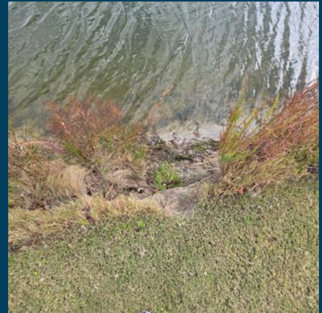
Lake Bank Erosion near lake #3
