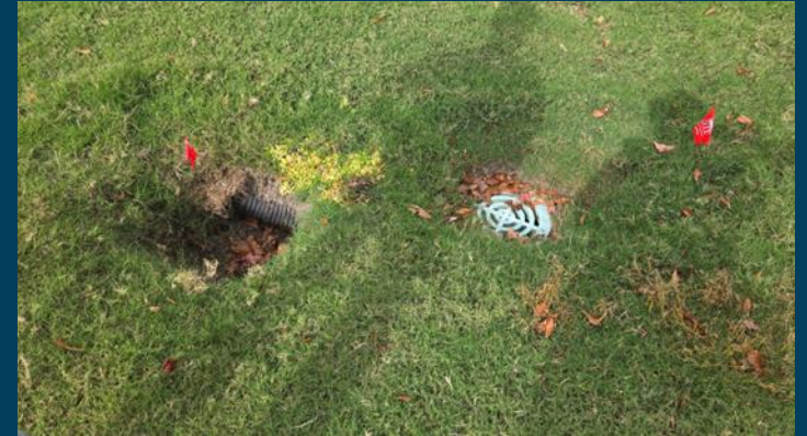
Sinkhole near the 6th green
